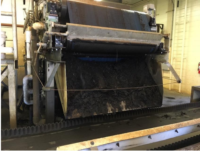
Figure WTR-3. Belt press used to dry WTRs at a smaller water treatment facility
